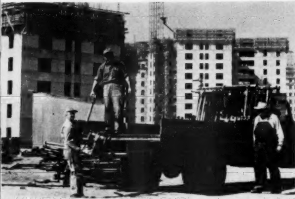
The big jobs, the small jobs—the plumbing, heating, air conditioning and appliance jobs in new construction, remodeling and improvement of residential, commercial, institutional and industrial buildings—are sold, installed, serviced and guaranteed by the domestic engineering contractor-dealer. He consults and plans with building owners, architects, and general contractors. He recommends and sells the products in his line.
